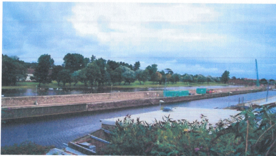
2016 Flood Defence Failure at former Bray Golf Club land
